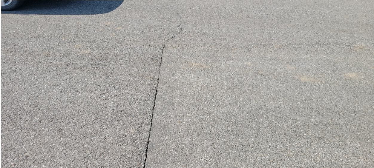
Figure 2: Longitudinal Joint Separation
